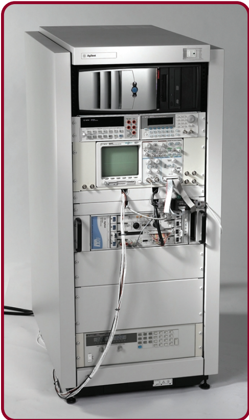
This test system was used to demonstrate the performance differences between USB, LAN, and GPIB interconnections to the Agilent 33220A function/pulse generator.
